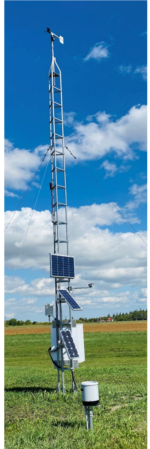
MB Ag Weather Station Installed in Arborg, MB
